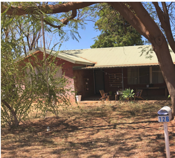
126 Cedar Street, Tom Price Full Refurbishment Required
