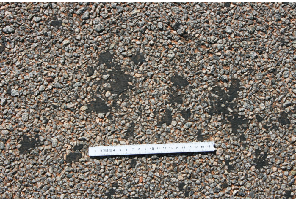
Figure 3.13: Apparent salt damage mitigated by pneumatic tyred rolling
