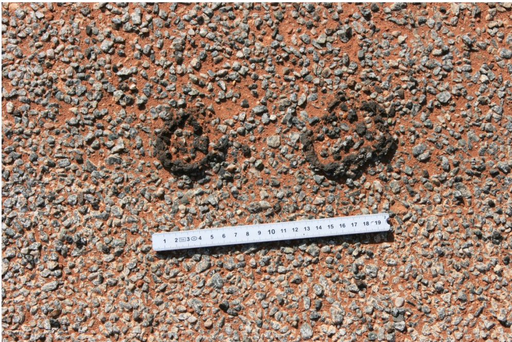
Figure 3.12: Salt damage on existing runway
