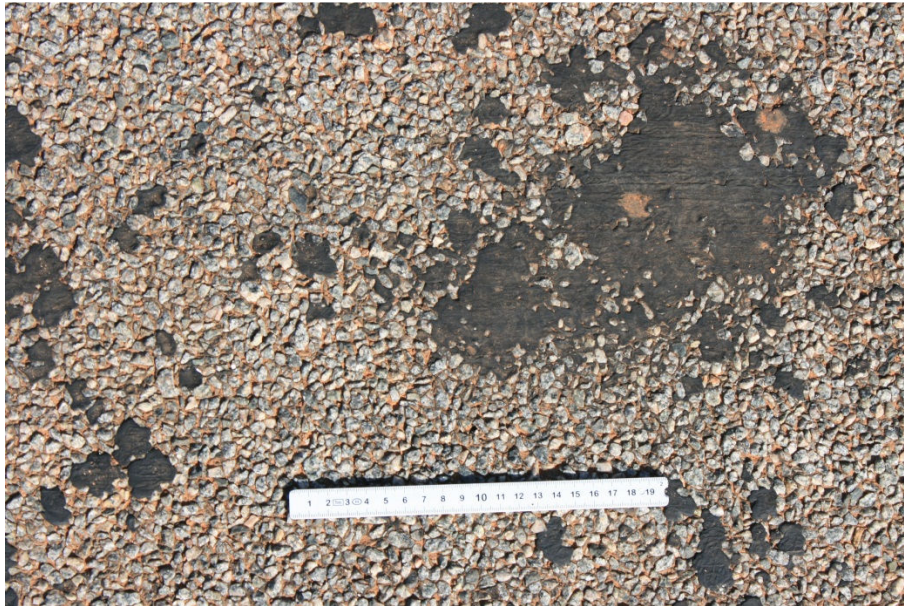
Figure 3.14: Apparent salt damage mitigated by pneumatic tyred rolling
