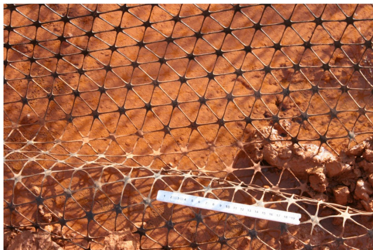
Figure 3.5: Tri-axle geogrid placed over natural surface prior to placement of select fill
