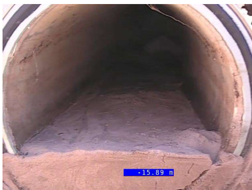
Chainage: ? - DES - Deposits - Fine sediment - 30-40%
