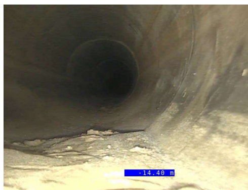
Chainage: ? - DEZ - Deposits - Other - 0-5%
