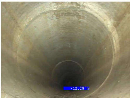
Chainage: ? - JDR - Displaced joint - Radial - 05-10mm
