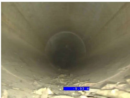
Chainage: ? - DEZ - Deposits - Other - 0-5%
