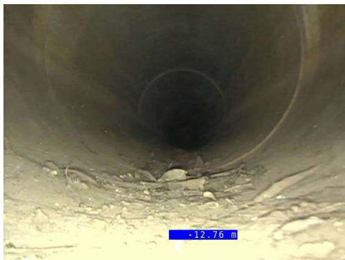
Chainage: ? - DEZ - Deposits - Other - 0-5%
