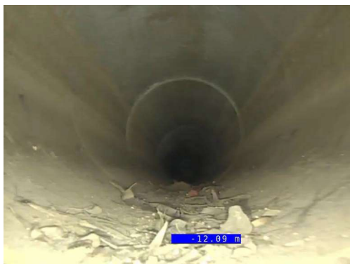
Chainage: ? - DEZ - Deposits - Other - 0-5%
