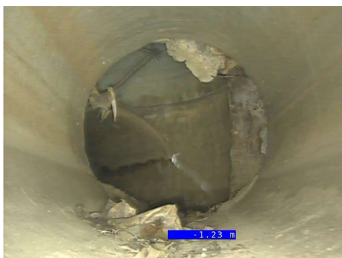
Chainage: 1.23 - DEZ - Deposits - Other - 0-5%
