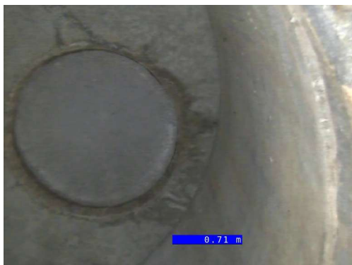
Chainage: 0.71 - FMMH - Finish node - Maintenance hole
