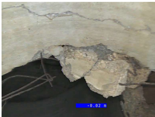
Chainage: 0.02 - BM - Breaking - Missing - 500-1000mm
