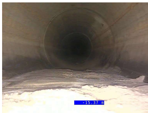
Chainage: ? - DEZ - Deposits - Other - 10-20%
