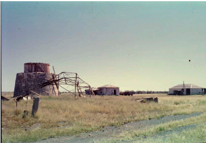
Left image: Water tank, 1885 dwelling and 1895 building after 1963 cyclone. Source: State Library of Western Australia 140132PD Right image: Water tank and 1885 dwelling 2016.
