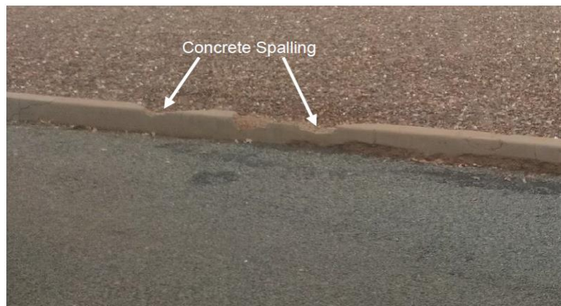
Figure 4. Concrete Spalling in Kerb – McRae Avenue, Paraburdoo
