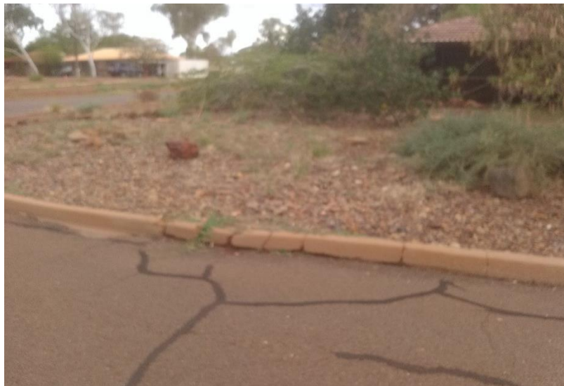
Figure 3. Cracked Kerb Requiring Replacement – Pepper Street, Tom Price
