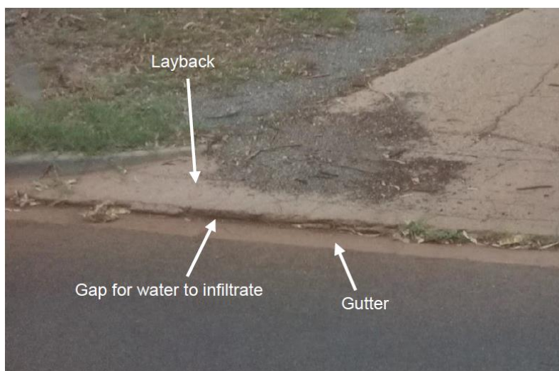
Figure 5. Vehicular Crossing Separating from Gutter
