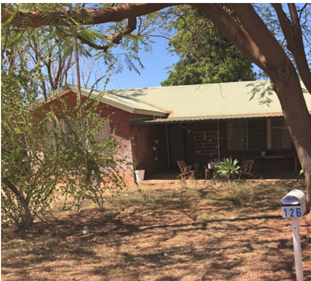
126 Cedar Street, Tom Price Full Refurbishment Required
