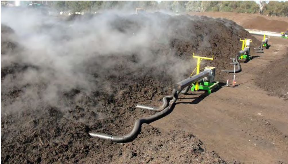
Plate 10-5: Mobile Aerated Floor composting system
