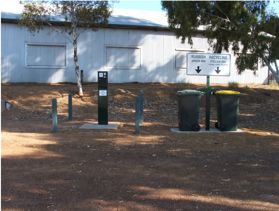
Coin operated meter providing potable water in Southern Cross.
