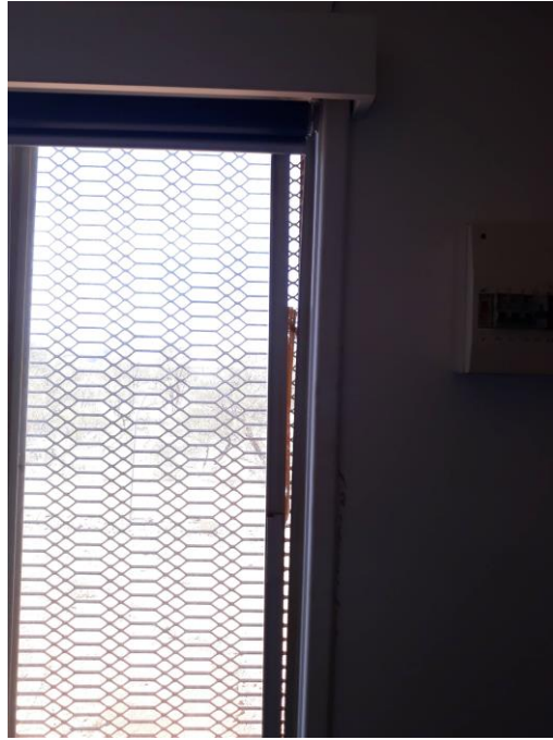
Figure 3. Misalignment of windows
