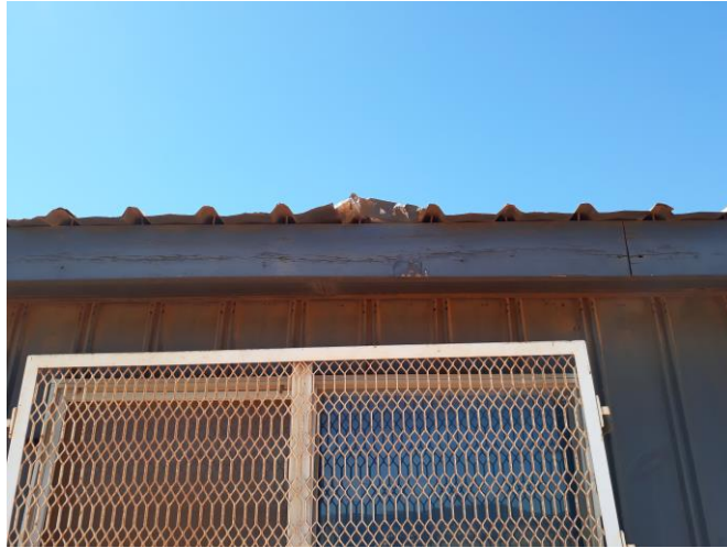
Figure 5. Damage to external cladding
