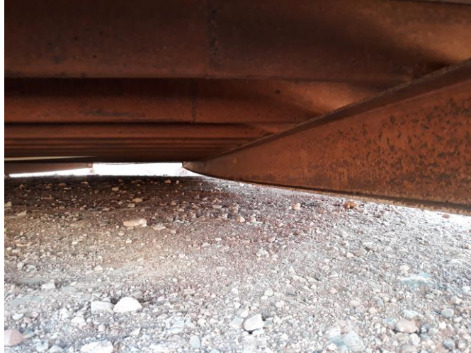
Figure 1. Structural beam with large deflection
