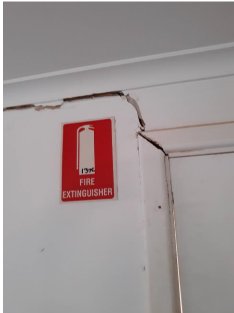
Figure 2. Cracking of internal plaster
