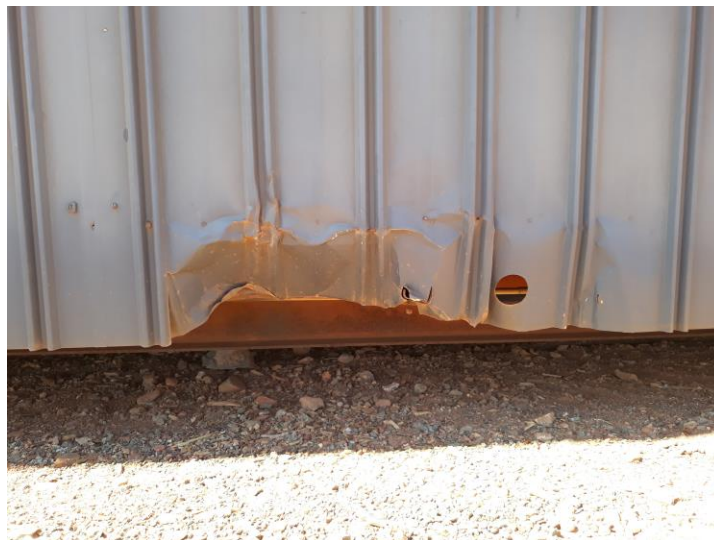
Figure 4. Damage to external cladding
