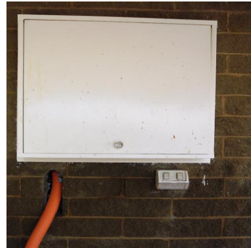
An entry point for the cable is made in the wall under the meter box
