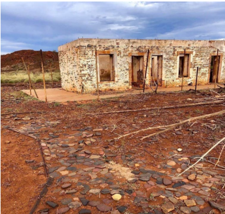
Figure 5 – Deepdale Homestead existing condition. Remnants of stone paths, verandah posts. Roof door and window joinery missing.
